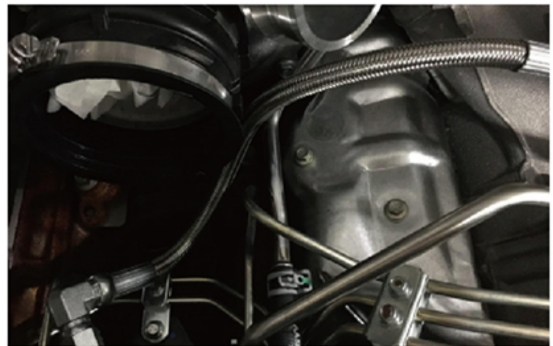
The line bracket that holds the supply and return hard lines is modified to allow attachment of the new braided stainless line by removing one of the "christmas tree" posts closest to the bracket mounting hole allowing the plastic snap to rotate and clear the braided stainless crimp collar. Top is unmodified bottom is modified. This is required for both versions of the kit. (pic page 11)
