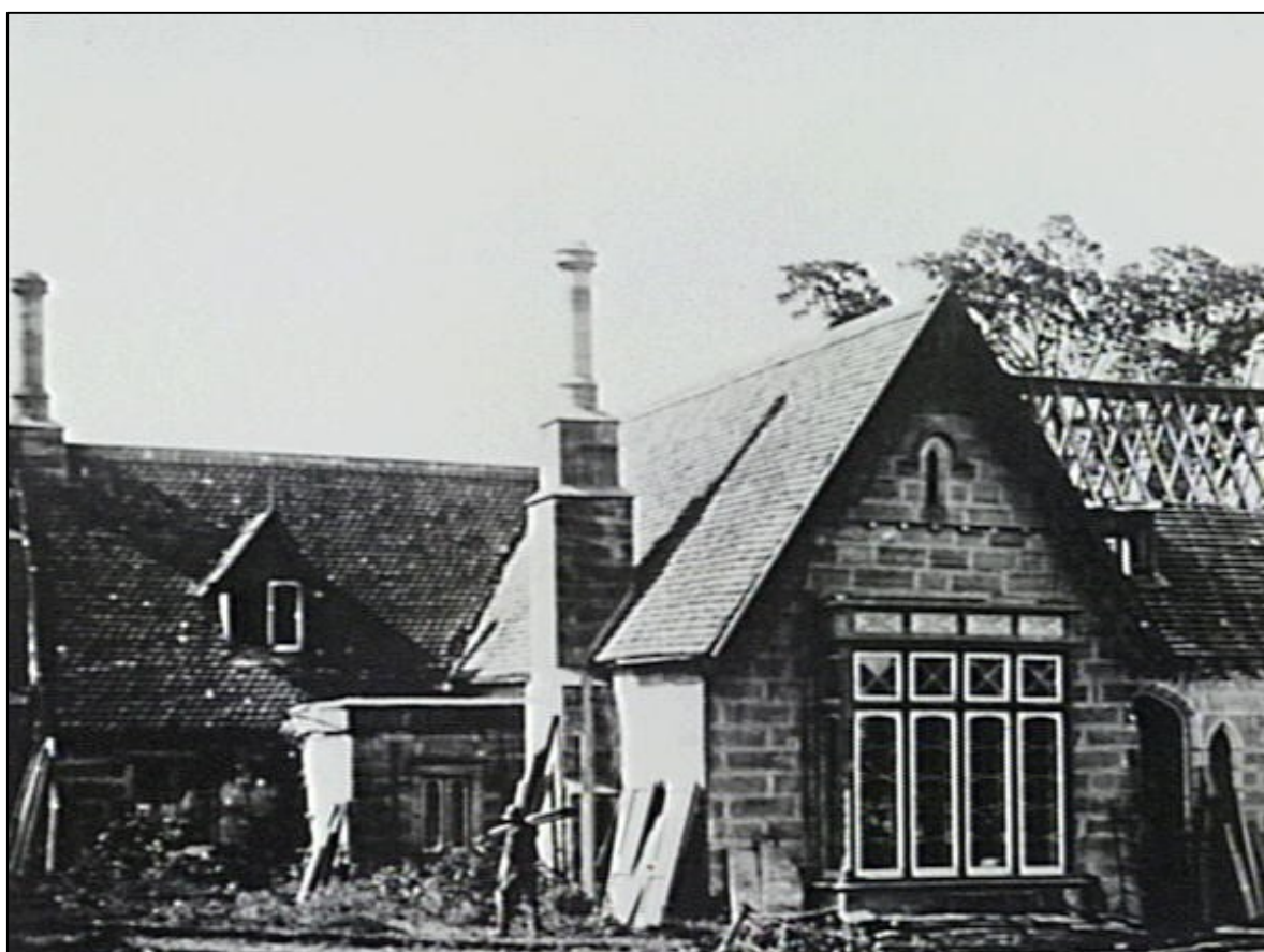
The roof being removed. The tiles were blue and red. (Ancher, p246)
