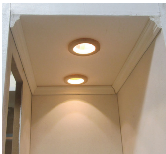
E225 Recessed Lighting
