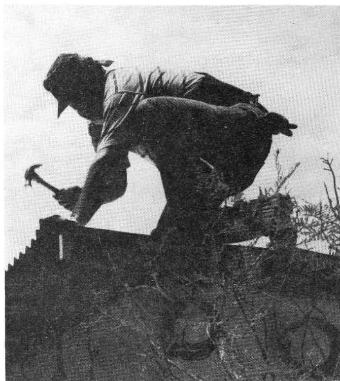
Within days of the closing, volunteers, work crews, and staff were busy filling dumpsters, clearing garden areas, and repairing the main house and annex. Here a roofer secures an edge of the new metal roof. Photo by Linda MacElwee
