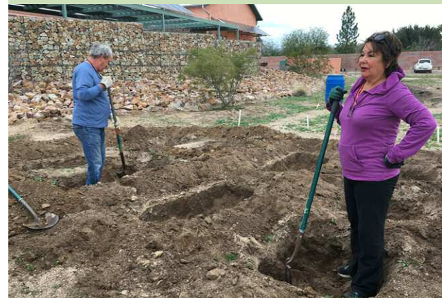
Volunteers Tom and Tatiana constructing Zuni waffle-style garden beds. The waffle design helps retain water.
