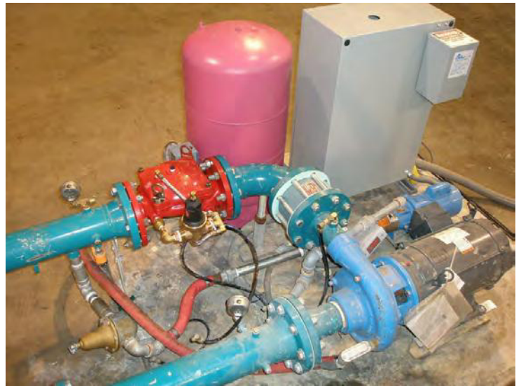
A constant pressure pump control valve working in conjunction with a VFD on a irrigation system.
