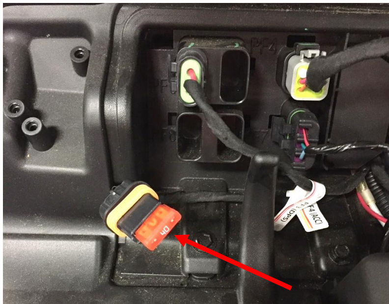
Figure 18: Factory fuse and fuse holder.
