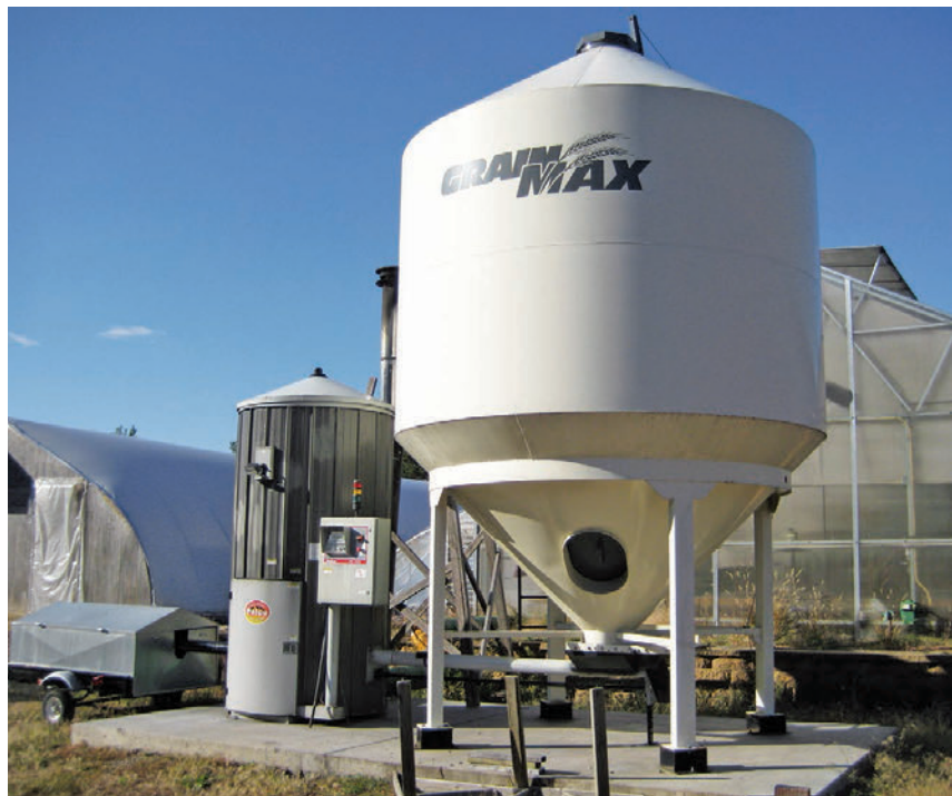
Hydronic pellet boiler with pellet storage bin.
