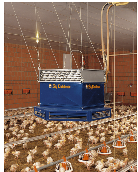
FIGURE 8. Hot water heat exchanger and fan. Photo courtesy of Big Dutchman, Inc.
