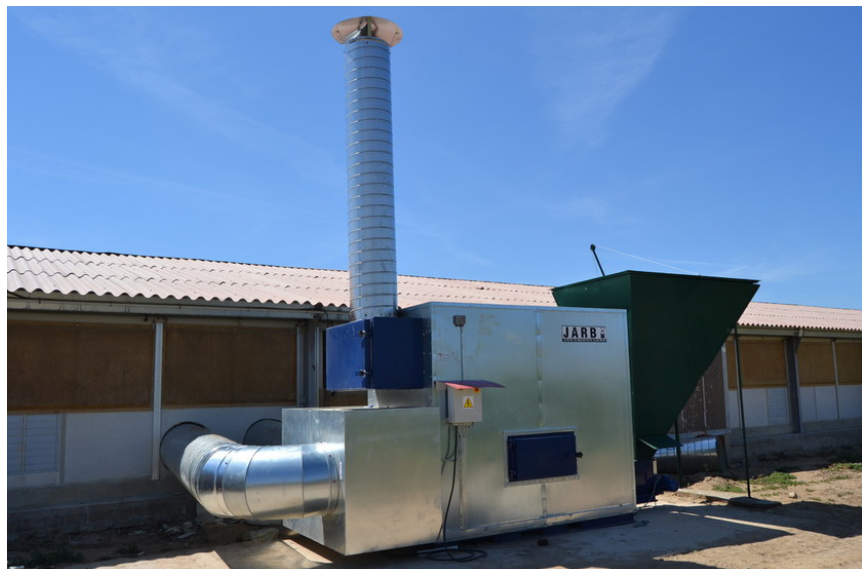
FIGURE 9. Wood pellet/chip furnace heating a poultry barn.
