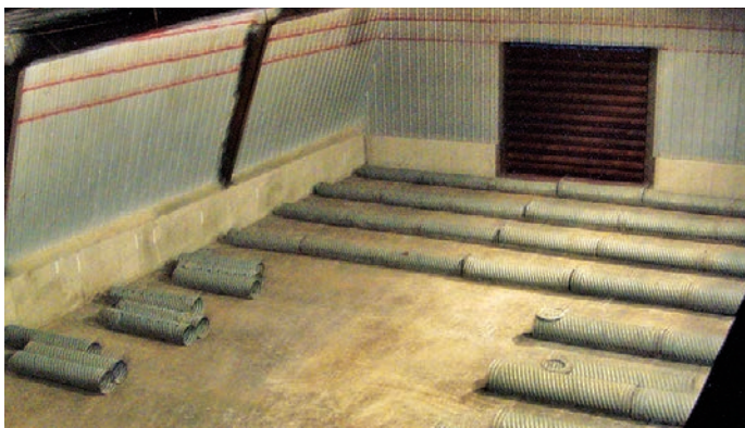
Figure 25. Potato storage with on-floor ventilation piping ready for new harvest. (Sanford)
