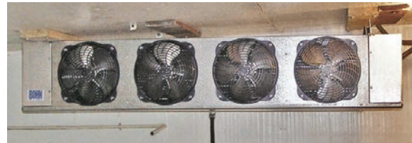
Figure 19. Ceiling-mounted evaporator units. (Sanford)
