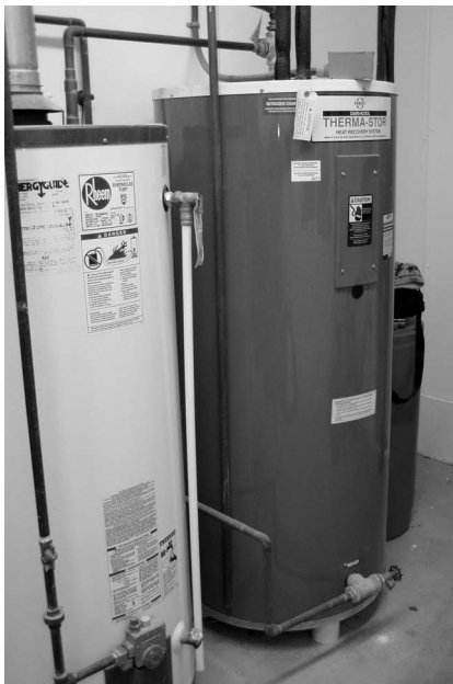
Figure 2. Typical refrigeration heat recovery installation next to water heater.
