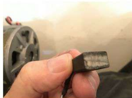
Before:: Needs cleaning & resurfacing with cleaning stone
