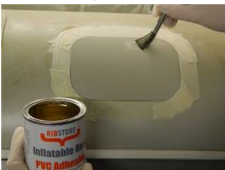
Applying the 2-part mixed adhesive to the masked and primed repair area
