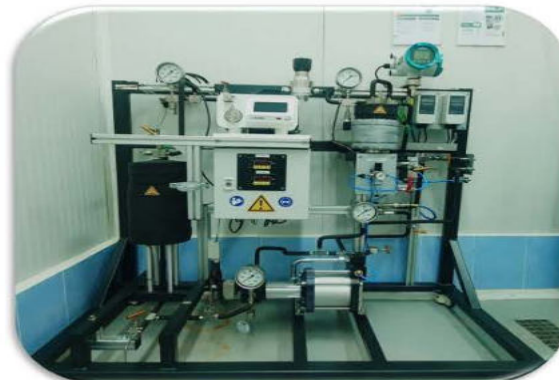
Supercritical CO2 plant
