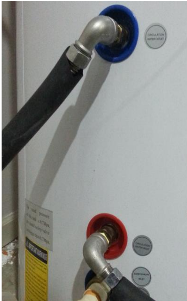
Elbows used on Solar Loop Connections to Tank to Prevent Thermo Siphon Effects
