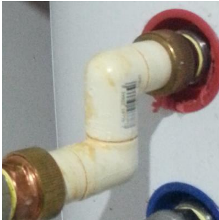
Hot Water Outlet with Elbow to Prevent Unnecessary Thermo Siphon
