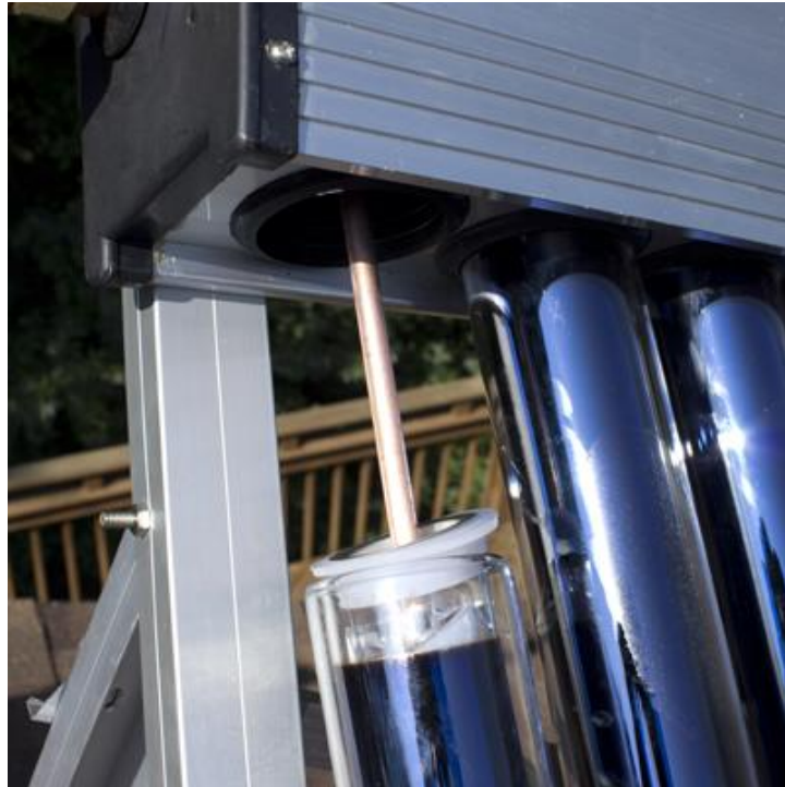
Pulling the copper heat pipe out of the tube so it can be pushed in by hand
