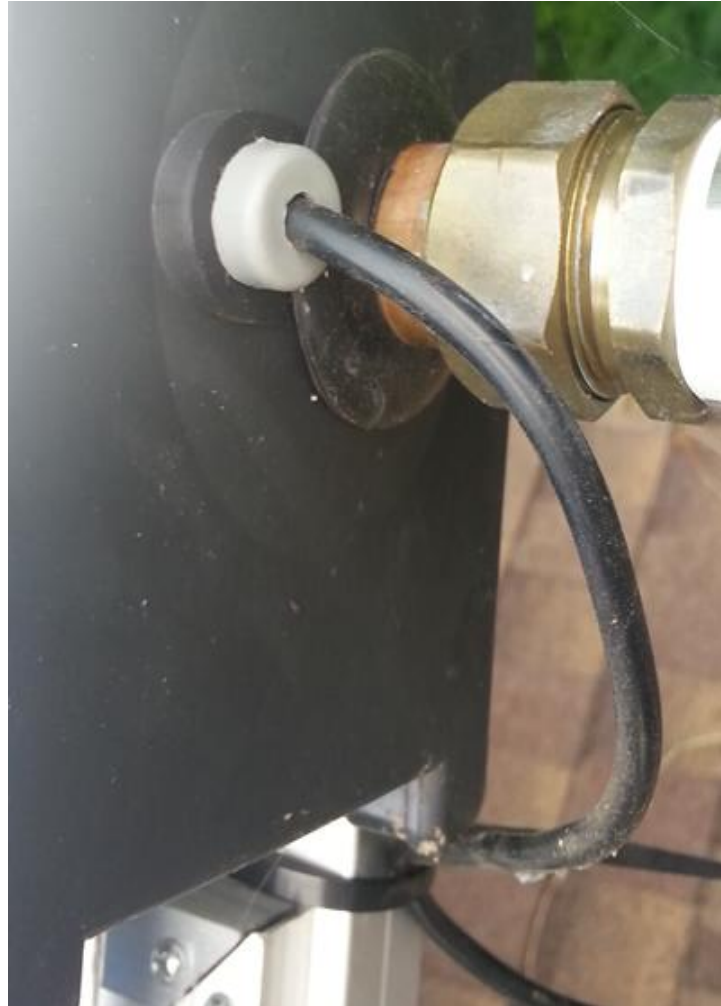
Properly Secured pt1000 sensor
