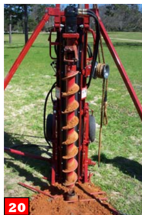
20 Loosen the (2) locking bolts. Raise drill head and remove hollow stem auger section.
