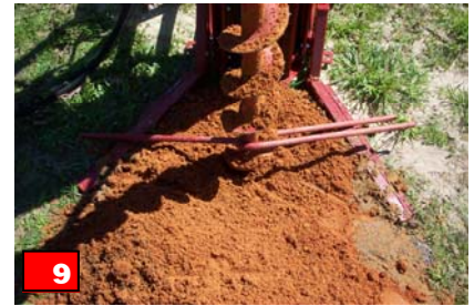
9 Once desired depth is reached, raise drill string to top of stroke. Insert auger fork (stop) around auger (extension) barrel approximately 6-8 inches below the top of the auger (extension).
