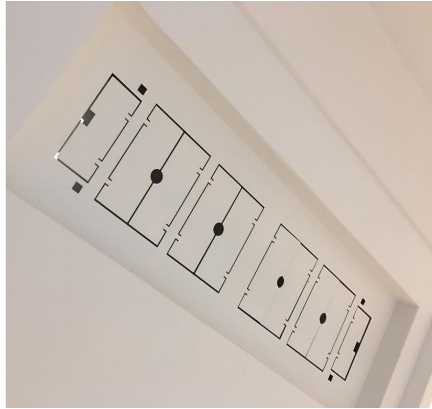
Above: Underside of air return, Drywall Pro Air Return, Project by: Jack and Greg Renovations, January 2019 - Toronto, Ontario
