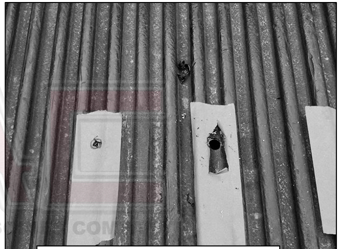
(Fig 2) First drill a pilot hole into the marked location, then use a 1/2inch drill bit to clear the 12mm T-Bolts
