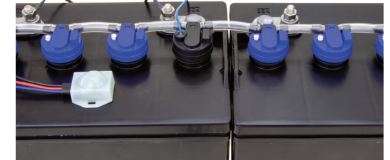
Installation with watering system
