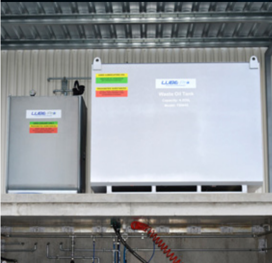
BULK OIL STORAGE SET UP CONTAINING A 4500L WASTE OIL TANK AND 1000L WASTE COOLANT TANK
