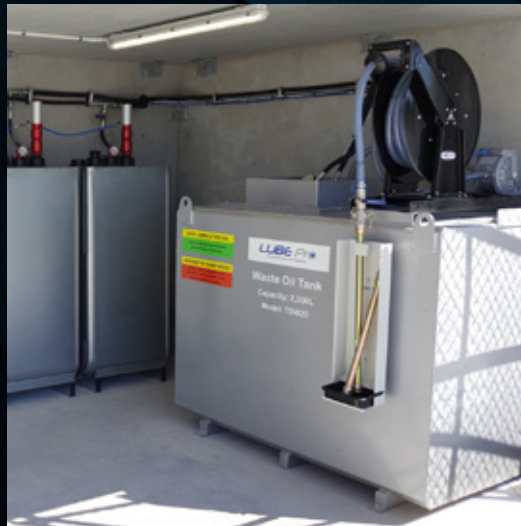
LUBE STORE WITH 2000L WASTE OIL TANK WITH MOUNTED SUCTION HOSE REEL AND PNEUMATIC WASTE OIL PUMP. TYPICALLY SUITED FOR SUCKING FROM MOBILE SERVICE VEHICLES
