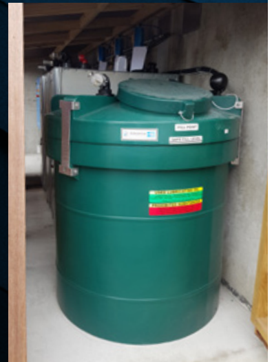
1000L PLASTIC WASTE OIL TANK WITH OUTER BUNDING TANK, INCORPORATED INTO TANK ROOM
