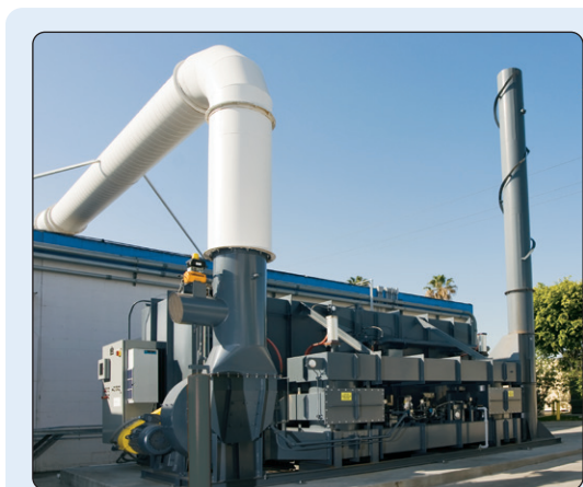
Our California facility takes pride in limiting volatile organic compound (VOC) emissions into the environment. Two regenerative thermo oxidizers are utilized to eliminate 99% of the VOC from our ventilation system before emitting air to the atmosphere.
