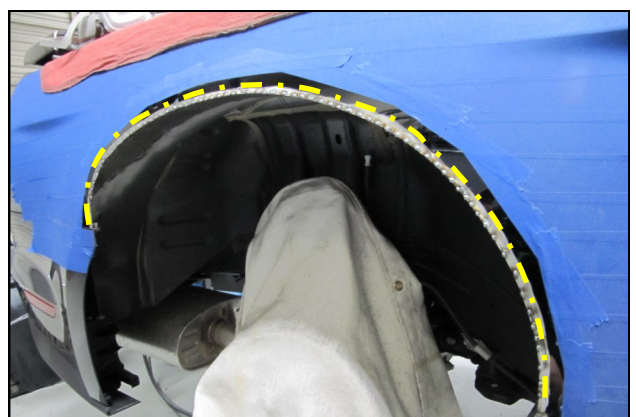
24. Continue tack welding along the inner and outer edges until sufficient coverage has been achieved.
