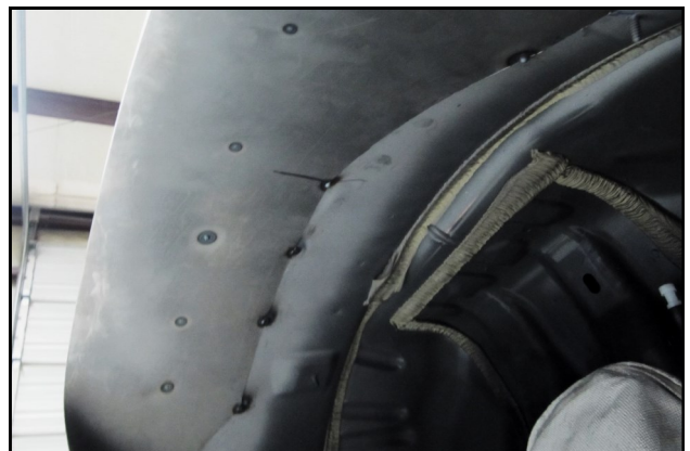
22. Alternate view of alternating tack welds. Use care not to overheat and warp the fender.
