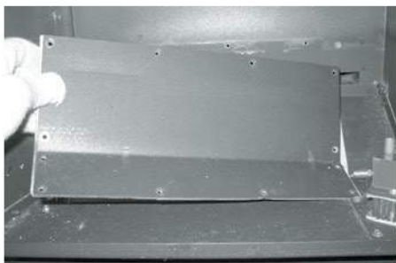
Fan Cover Plate Removed
