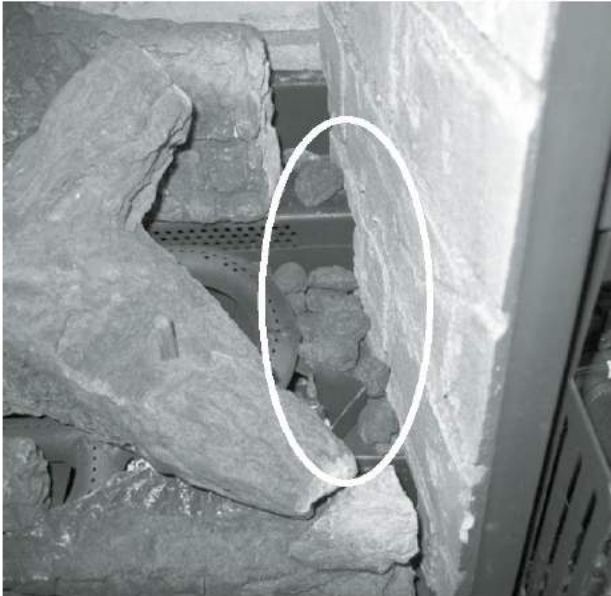
Right side of Burner
