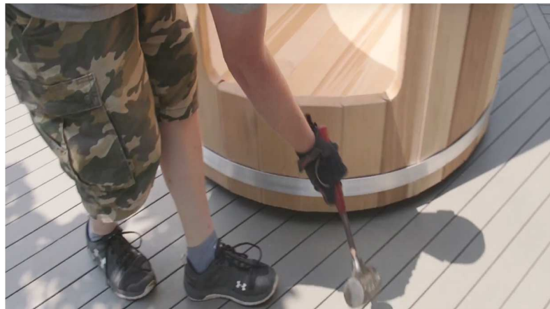
28. Work around the shower, hitting each stave with a firm tap right on the bottom strap. You will see each stave sit a little tighter.
