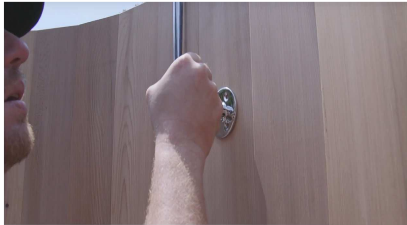
31. Line up the shower head assembly with the stave that has the holes.
