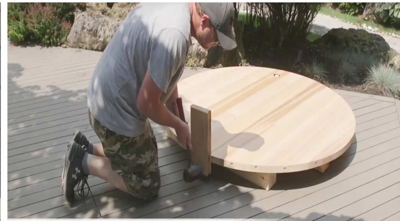
10. Attach bottom entrance staves on the opposite side from the floor drain.
