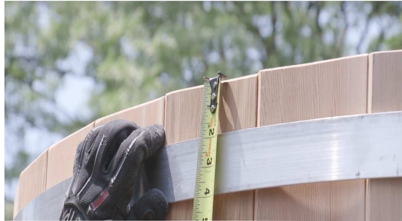
26. Make sure the metal bands are 2" from the top and bottom all the way around the shower.
