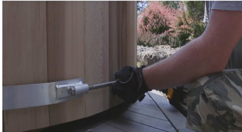
27. Using a wrench or impact driver tighten each band a little at a time, starting with the bottom. Tighten the band in stages-bottom first then top.
