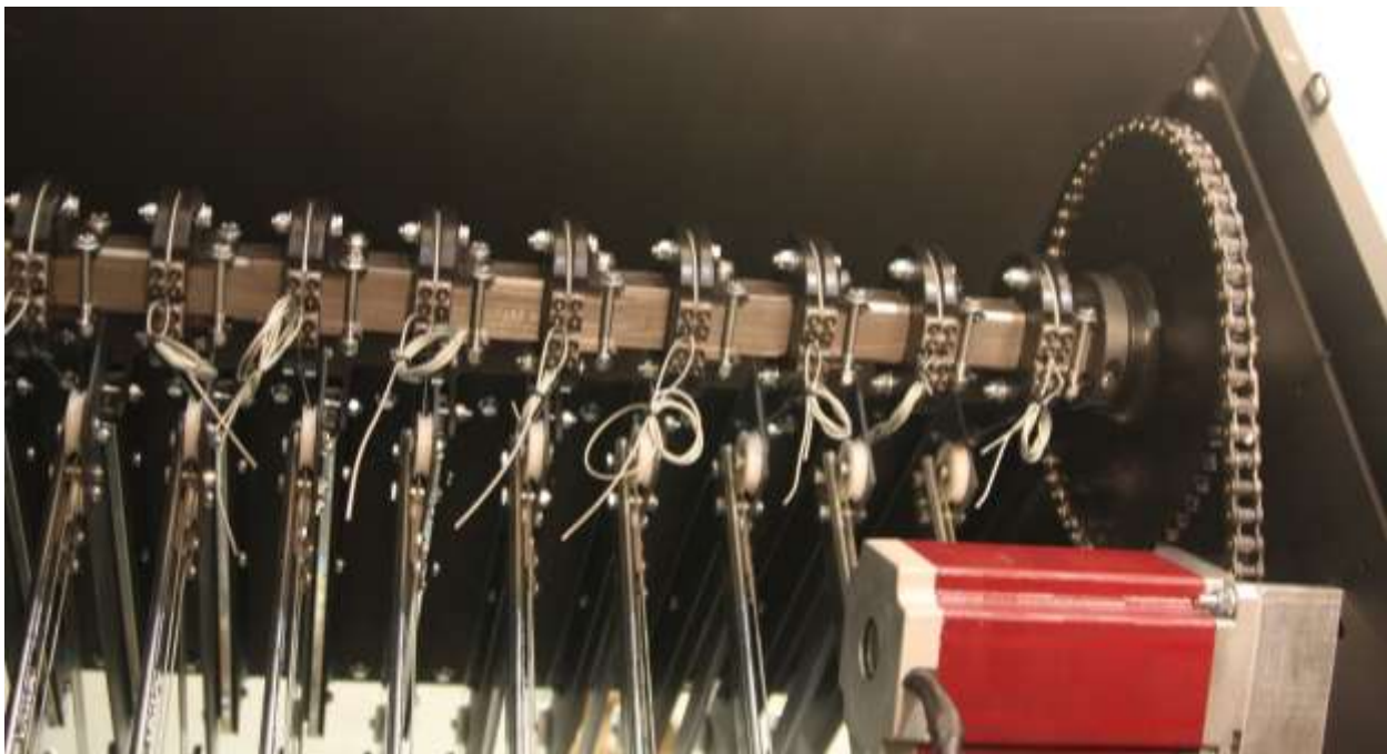
Drive Chain (Inside Control Box)
