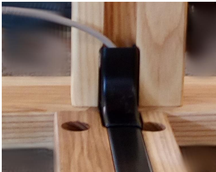
Figure 10 - Connection Cover on loom
