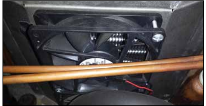
Figure 6-13. Condenser Fan Motor/Fastener
