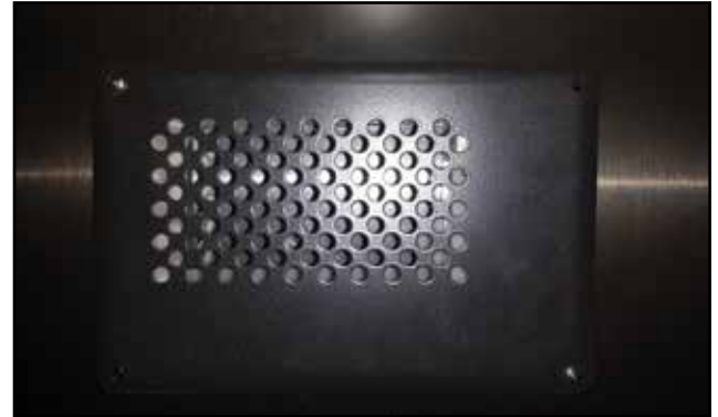
Figure 6-5.2. Evaporator Air Damper Outlet Openings
