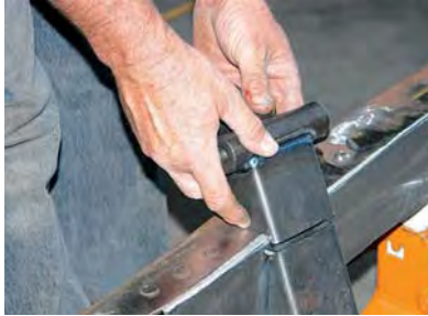
11) The upper A-arm mount or tower had to be installed next. It was placed on the frame and extends upward from the lower crossmember.
