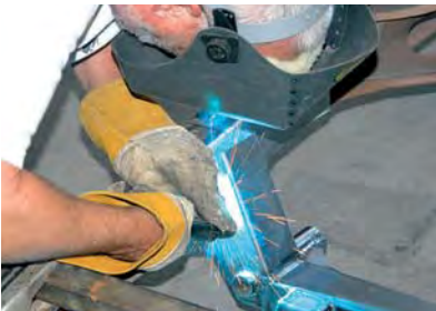
10) After all of the measurements were made and the crossmember was located correctly, it was tack-welded to the frame.
