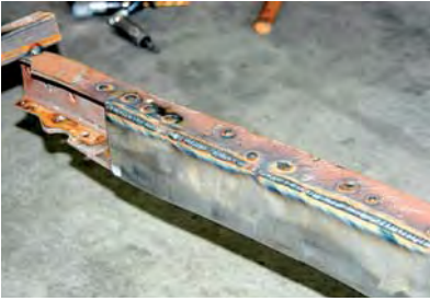
7) Here's what the framerail looked like after it was boxed. This strengthens the frame at the point where the crossmember will be installed. Without this, the frame could tear from stress over time.
