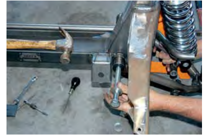
15) The lower A-arm was installed using the long bolt supplied in the kit. Washers are supplied to rest against the urethane bushings.
