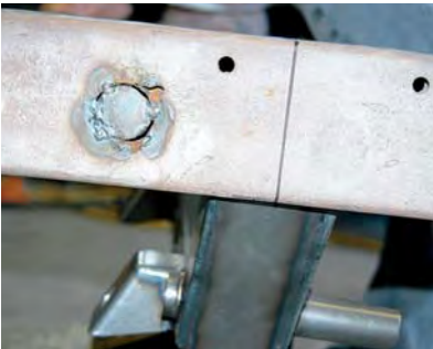
9) Here's the centerline on the frame lined up with the centerline on the crossmember.
