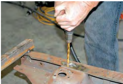
2) Using a 3/8-inch drill, the rivets were drilled to remove the shanks.
