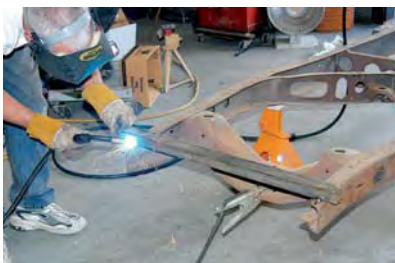
1) A heavy-wall-thickness square tube was tack-welded to the chassis to hold it in place when the stock crossmember is removed.
