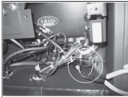
Figure 1 Jumper wire disconnected
