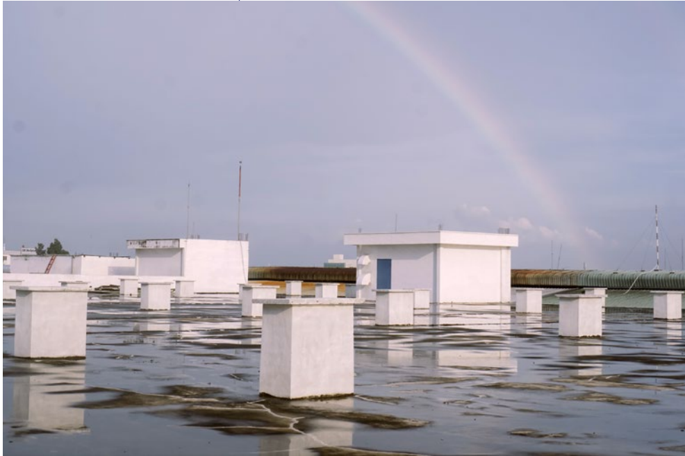
The roof of our Sài Gòn factory, where in the future we plan to install solar panels.
