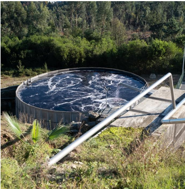
Figure 7: Water treatment plant at one of the dyehouses in our supply chain
