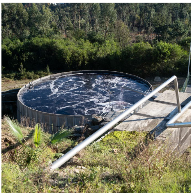
Figure 7: Water treatment plant at one of the dyehouses in our supply chain
