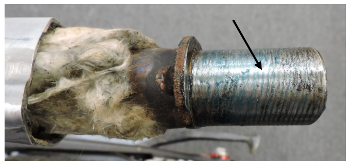
Figure 4 -Black arrow identifies cleaned & greased portion of exhaust tube.
