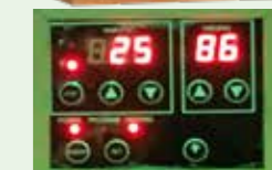
Fig 1. POWER & HEATING lights illuminated to show sauna in operation
