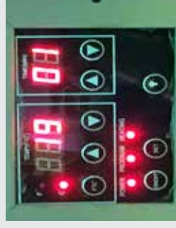
Fig 3. Three lights will indicate the sauna is heating
