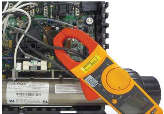
WHEN TESTING AMPERAGE
