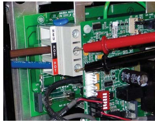
Brown to Blue Wires on a 230V BP600 System
