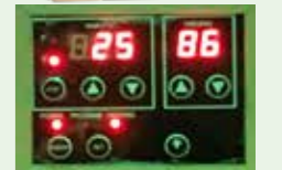
Fig 1. POWER & HEATING lights illuminated to show sauna in operation
