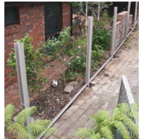
Set all the bottom rails into position ensuring a 50mm ground clearance.
