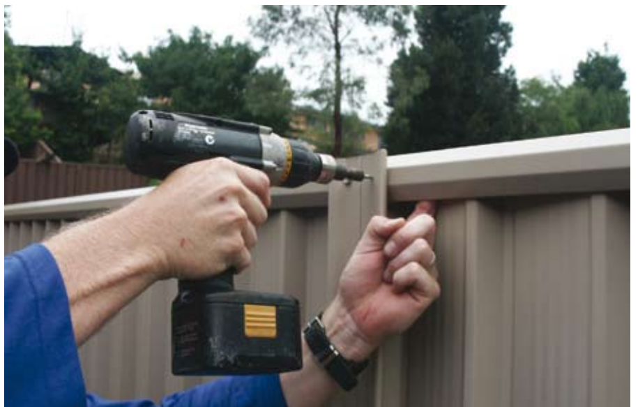
Screw off top rail and make it as close to parallel with the bottom rail as possible. Stand back and look at your work as you go along.
