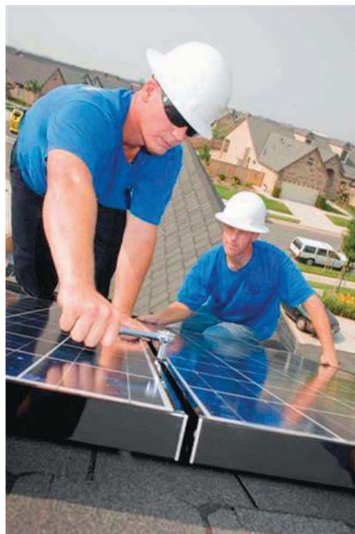
Check all bolts
