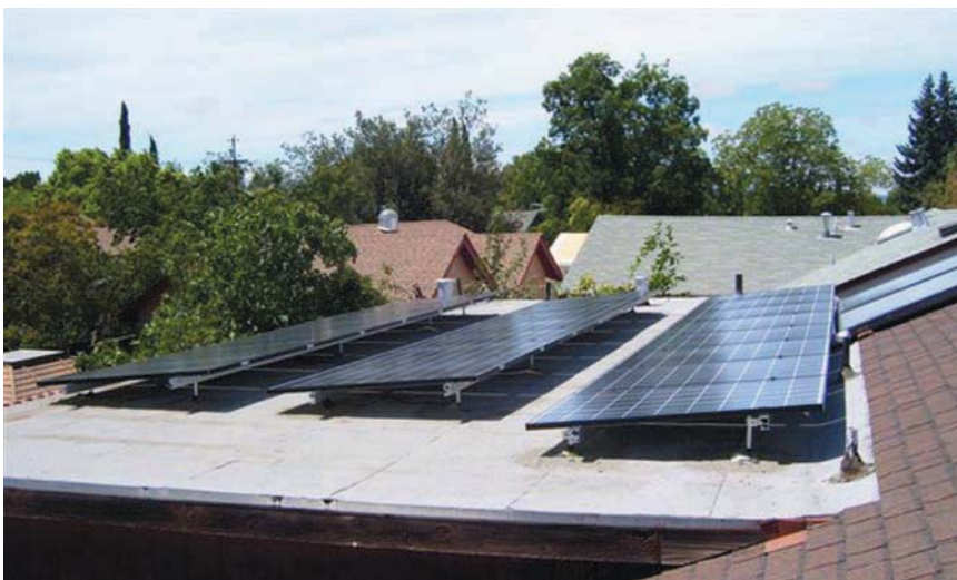
PV modules installed at shallow angle
