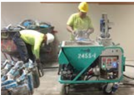
Commercial Flooring from Cold Spring, NY using the Koine 35 for laying down thousands of bags of self-leveling underlayment in West Point Military Academy, West Point, NY.
