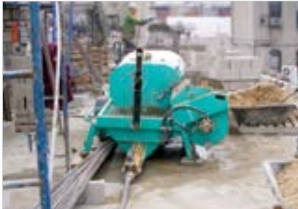
Concrete block walls are being filled with the Silent 300 which is shown with the optional larger 60.12 rotor/stator. Notice the grout is being made the old time way – shovels of sand and some portland.
