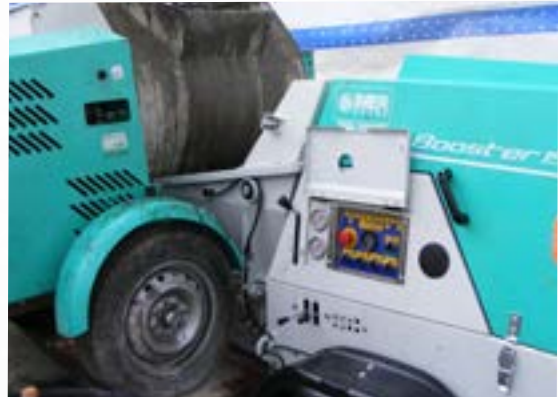
Conti Construction using the Booster 15 for pumping Sikacrete 211 while being fed by a mixer up to the Whitesone bridge in NYC.
