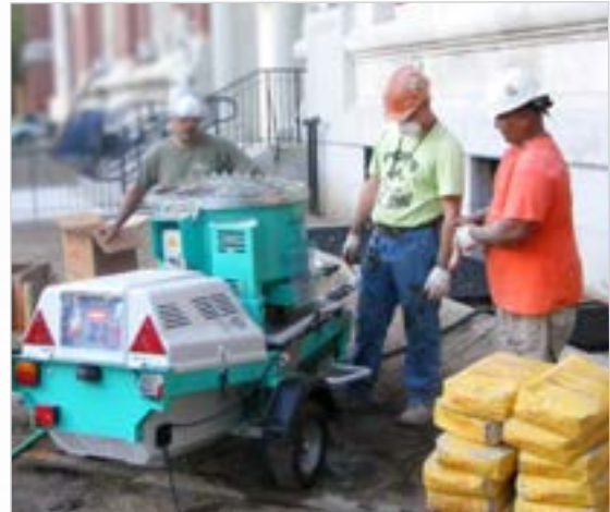
The Step-Up 120 shown above was used to mix and then pump Sika grout with the addition of small aggregate into a broiler room 200 feet away. This was a public school job and the grout was used to fill forms and encase the structural steel beams.
