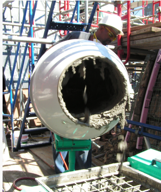
Minuteman being used on the top of the Plaza Hotel in NYC. Feeding into the Mighty Small 50 for shotcreting the dome repair.
