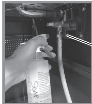
GAS HOSE COUPLING CONNECTION AT FIRE TABLE GAS VALVE
