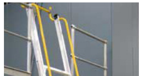
A Safety Gate is provided at the upper floor level to maintain the integrity of the perimeter railing.
