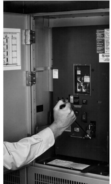
Two-Step Stored-Energy Closing
