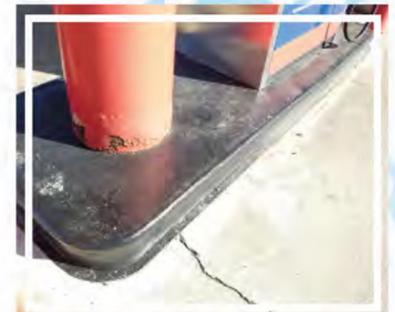
Rusty Canopy Supports
