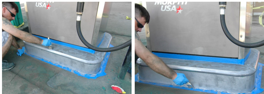
STEP 3B REINFORCE THE TYPICAL RUSTY AREA WITH MORE RUST ARMOR PRIMER—THE TOP PERIMETER OF METAL CURB AND THE BOTTOM OF METAL CURB.
