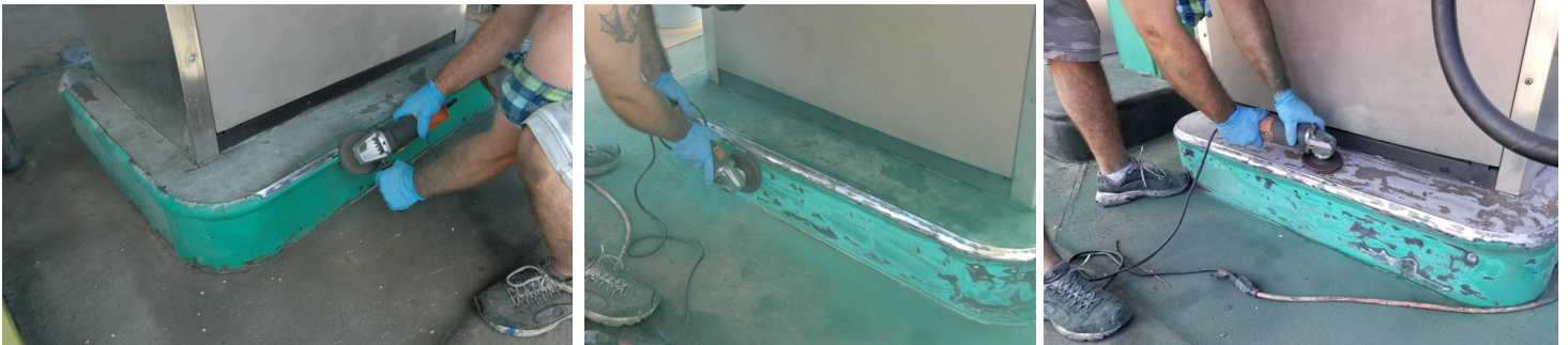
STEP 1 GRIND LOOSE PAINT AND RUSTY METAL WITH AN ABRASIVE GRINDING DISK.
