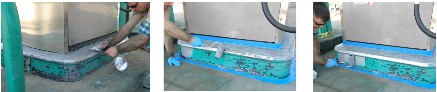
STEP 2 SOLVENT WIPE CONCRETE AND METAL CURB. THEN WIPE METAL WITH A METAL CLEANER / RUST CONVERTOR.
