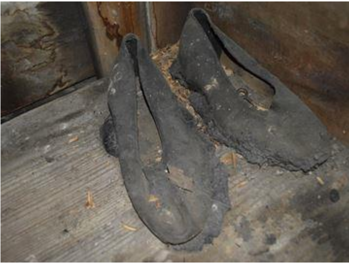
A pair of old shoes sit stuck in tar in a cubby on the way to the roof of the old Odd Fellows building.
