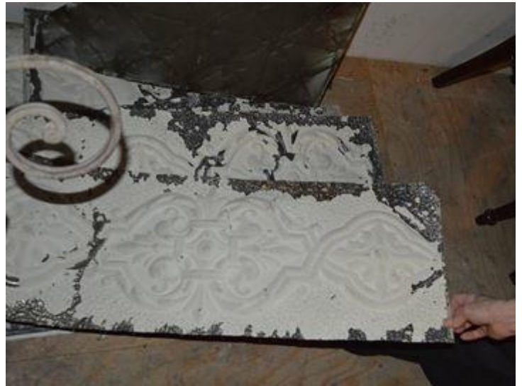
Tin tiles from the ceiling were in need of straightening and a fresh coat of paint when Elise Boyer bought the building from the Odd Fellows.
