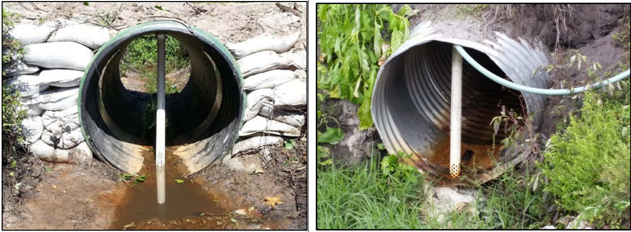
Figure 8 -Typical surface water collection within seepage ditch (left) and culvert (right). Autosampler intake tube, temperature and conductivity probes are located within PCV pipe attached via hinge to top of culvert to allow high flow events.
