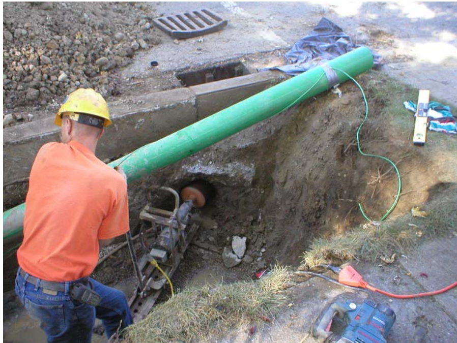
Figure 8-5. Curb drains convey disconnected footing drain flow to the storm water system.
